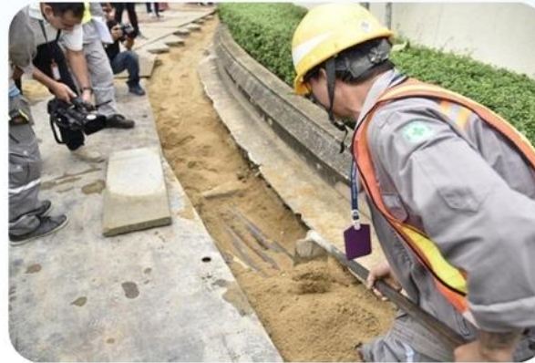
PEA Underground Cable Systems (Phuket, Phitsanulok)
